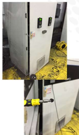
Magnetic dust found inside drive enclosure
