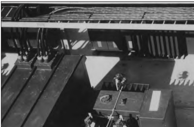
Cables Exiting 480 Volt Outdoor Switchgear and Entering Cable Tray System (Cable fittings with clamping glands are required to prevent moisture flow into equipment due to the cable's overhead entry into the switchgear enclosure).
